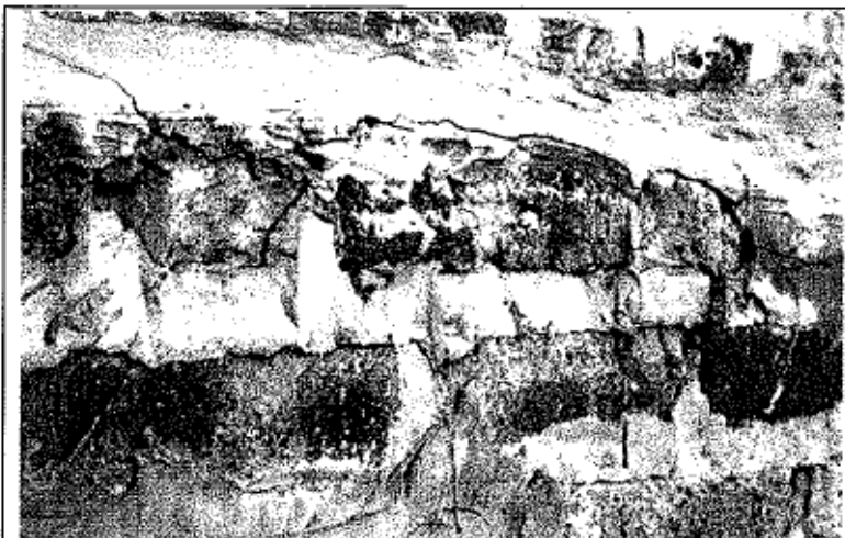
Figure 7. North elevation parapet wall. Cracked, loose and weathered mortar joints.
