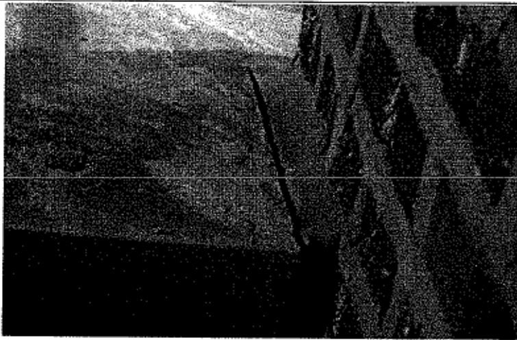
Figure 18. Opened and non-bonding sealant joints around limestone joint.
