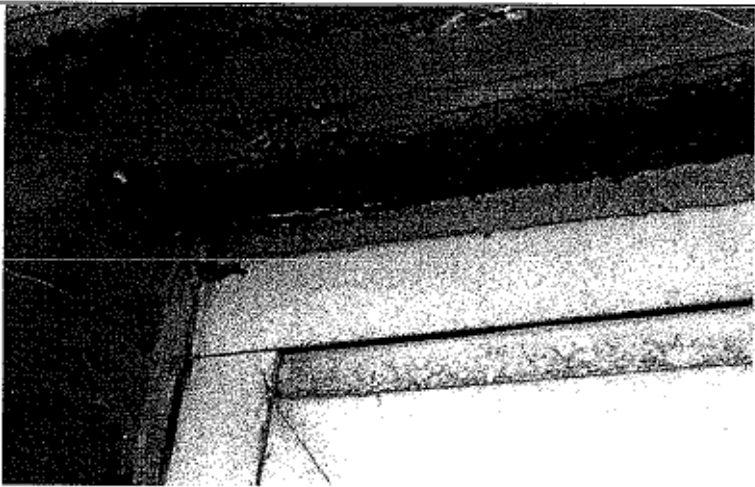
Figure 10. Corroded steel shelf angle at the top floor on the east elevation. Previously painted shelf angle is deteriorating, the result of no flashing details.
